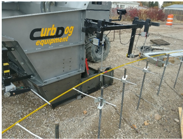
Figure 5. When using a fiberglass rod as a guideline for radius work, increase stake spacings. But make sure the transition between the rod and stringline is properly set.
